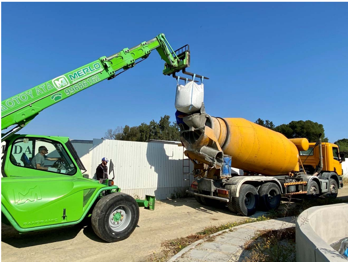
Figure 1. Addition of Recycled Concrete Aggregates (RCA) in concrete truck mixer for treatment.
